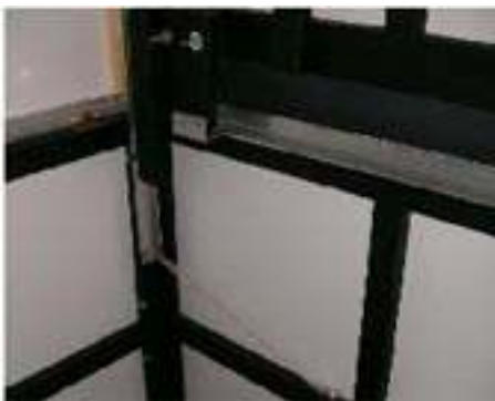
The image below shows the other side of the mechanism with a piece of 'bungie' to help the door stay in contact with the guide wheel when the door is lowered.
