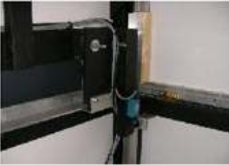
Image above shows the mechanism that closes the door and the closed limit switch. One of the roof safety brackets can also be seen. Four of these are installed to prevent the roof from lifting during high winds if the roof happened to stay open during failure of the wind sensor.
