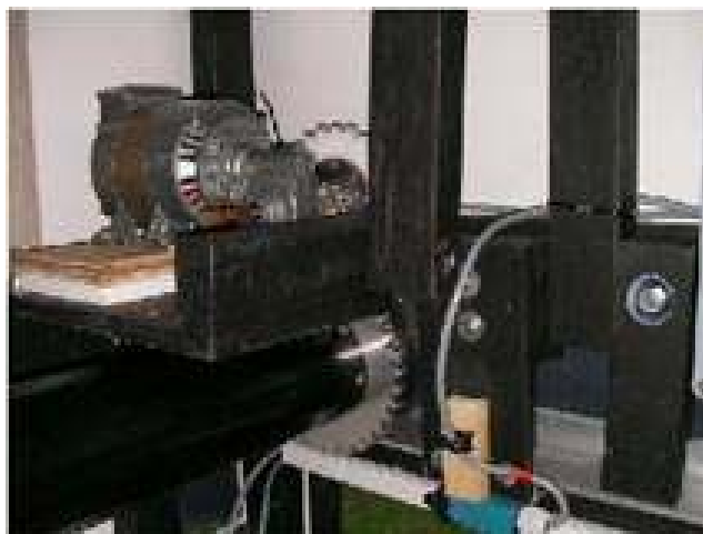
The image above shows the new motor in place (some painting is
